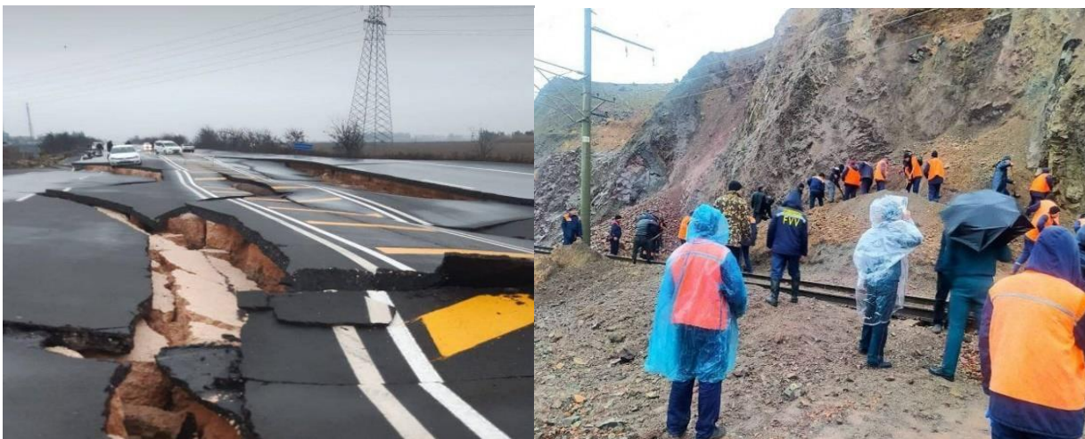
Figure 1. Primary and secondary damages to roads and railways caused by earthquakes.
